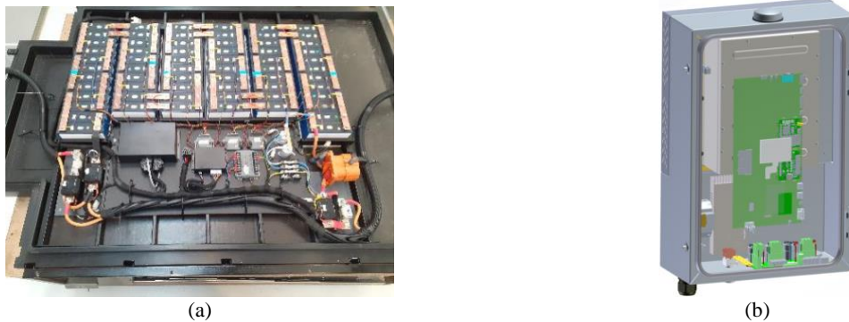
Fig. 9. (a) LFP prismatic cells in a 100 V configuration; (b) 7 kW DC wall box charger, with front door removed.
